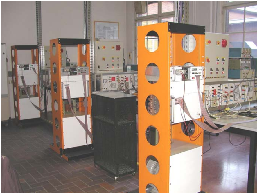
Figure: Practical setup of Herakles platform with 3 power electronic converters, interconnected via a TCP/IP based info'structure.
